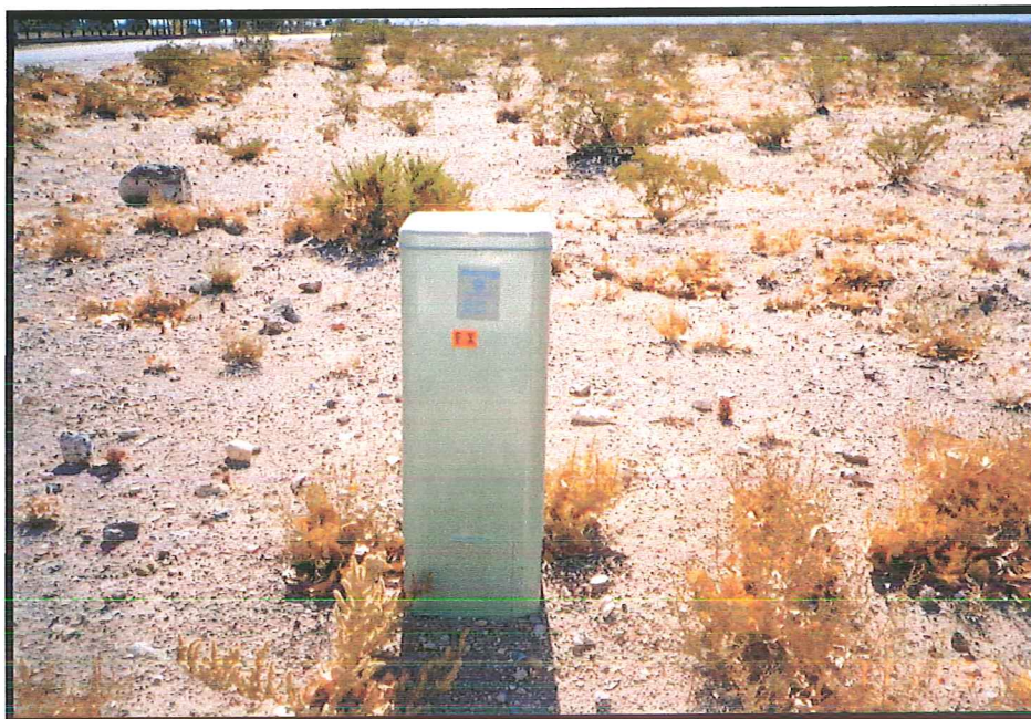
Photograph 8: View of the fiber optic box located at the northeast corner of the property.
