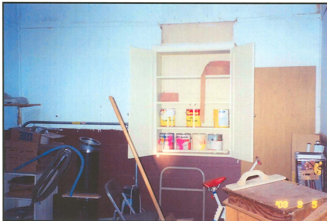
Photograph 8: View of paint containers and fluorescent lights in storage room.
