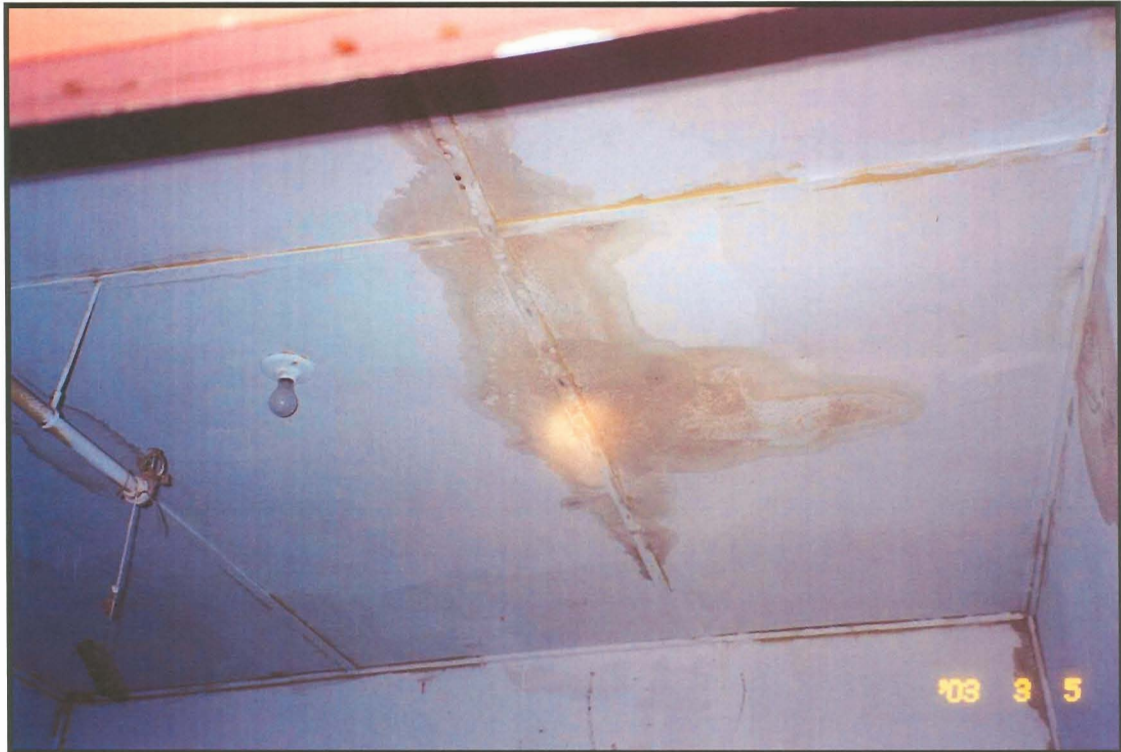
Photograph 3: View of water marks from leaking ceiling.
