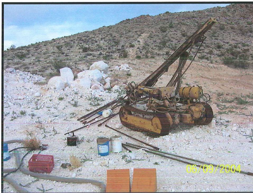
Photograph 6: View of boring equipment and containers of lubricating oil at borrow pit on Section 16, facing northeast.
