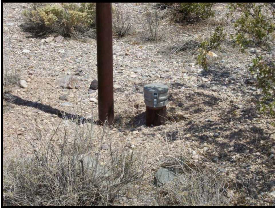
Photograph 11: View of fill port at base of vent pipe associated with fuel pump on subject parcel 018-021-02, facing west.
