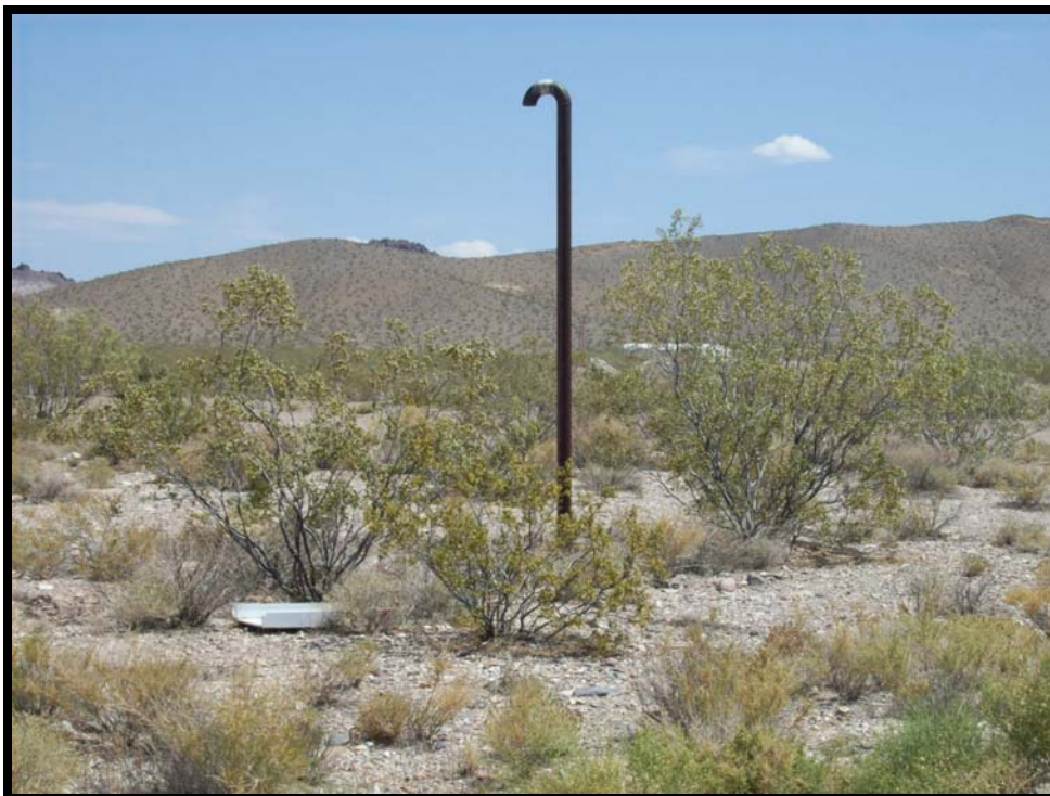
Photograph 10: View of vent pipe associated with fuel pump and UST on subject parcel 018-021-02, facing west.
