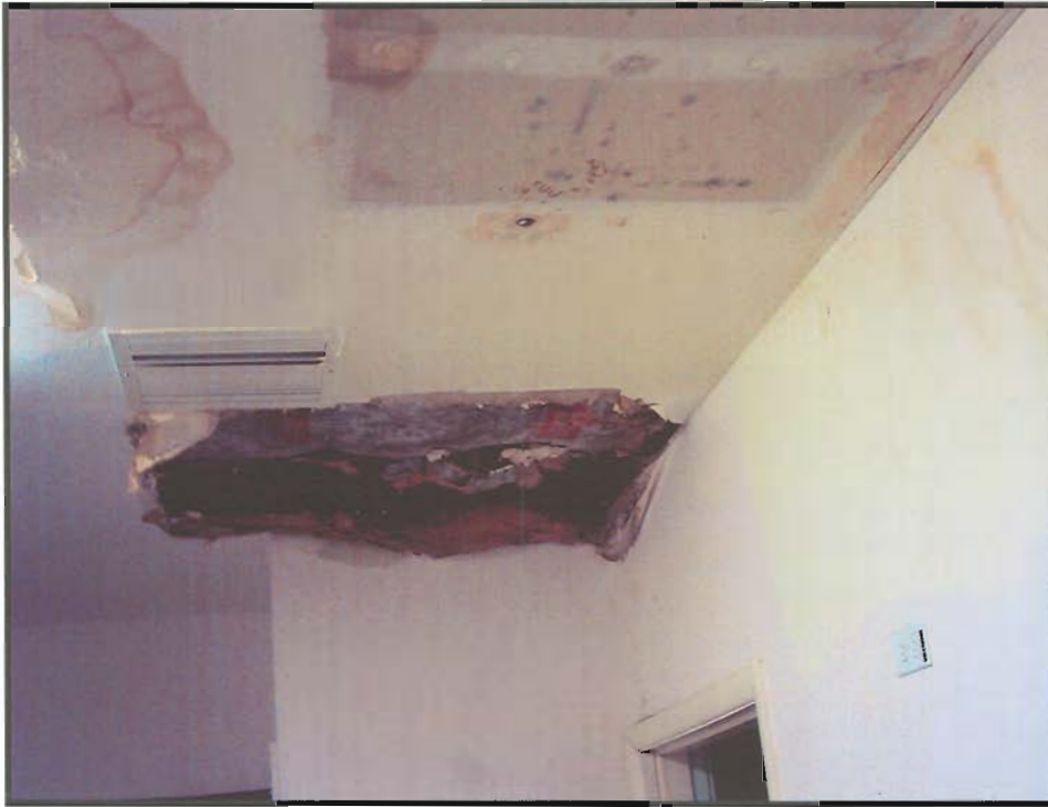
Photograph 7: View of water intrusion areas and associated visible mold within the main building.
