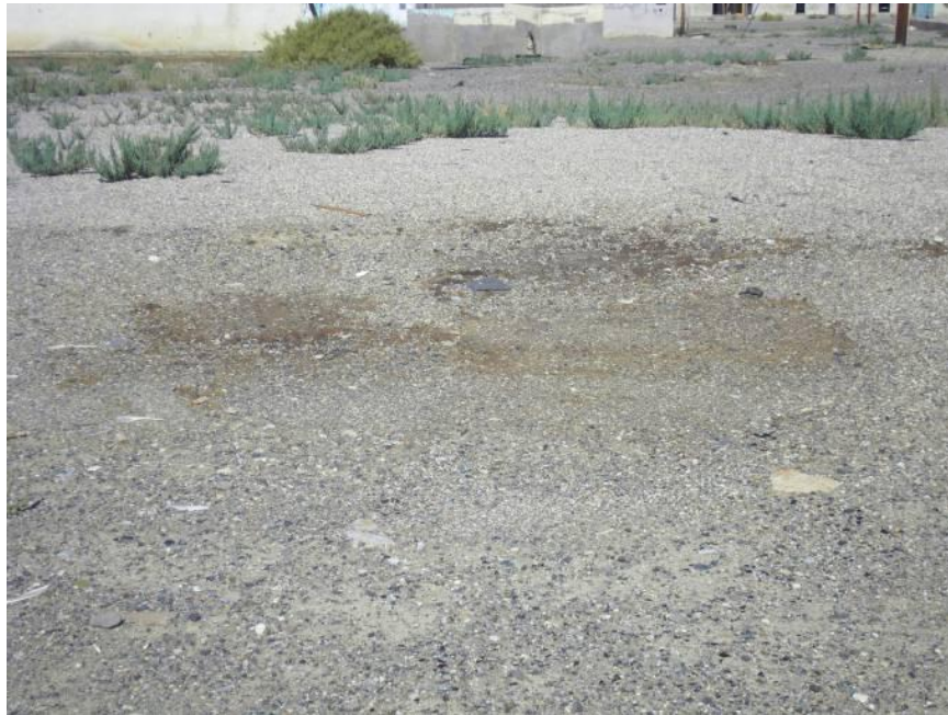
Picture 45. Close up view of surface staining in the location of the former above-ground storage tanks.
