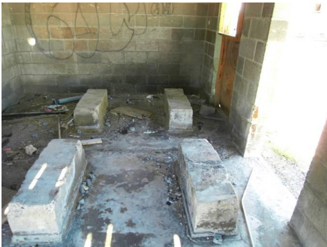
Picture 13. Additional interior view of diesel generator room.
