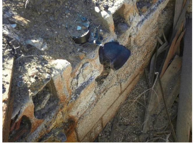
Picture 30. Another view of the former on-site septic system (note piping in middle).
