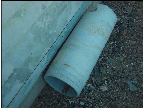
Photograph 17: Suspected transite pipe on the along northwest exterior of Building 7, Motel Units.
