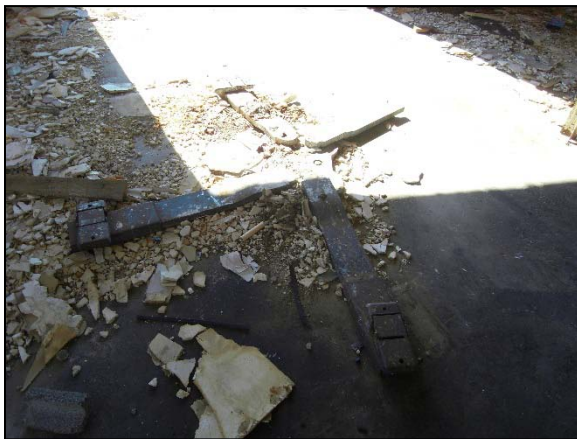
Photograph 3: Hydraulic Lift in Building 1, Former Service Garage (looking east).
