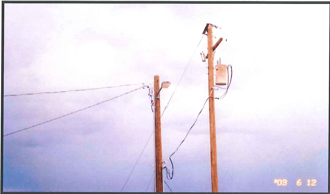
Photograph 7: Pole mounted transformer centrally located on the subject site.
