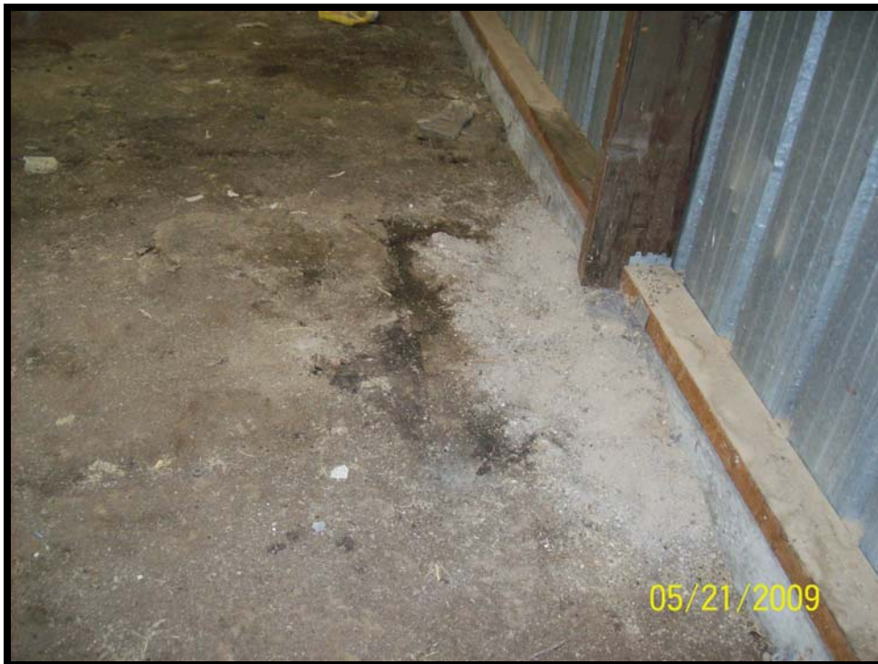
Photograph 9: View of stained soil inside hangar.
