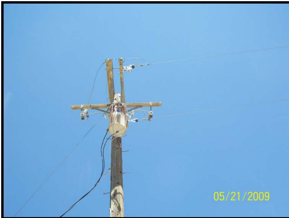
Photograph 13: View of pole-mounted transformer on southeast portion of site.
