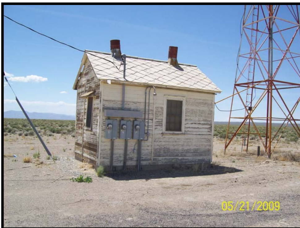
Photograph 12: View of beacon tower and associated electrical building on southeast portion of site, facing southwest.
