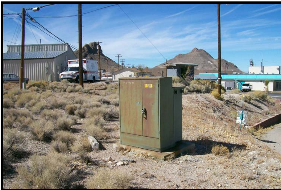
Photograph 14: View of electrical box on northern margin of subject site, facing west.
