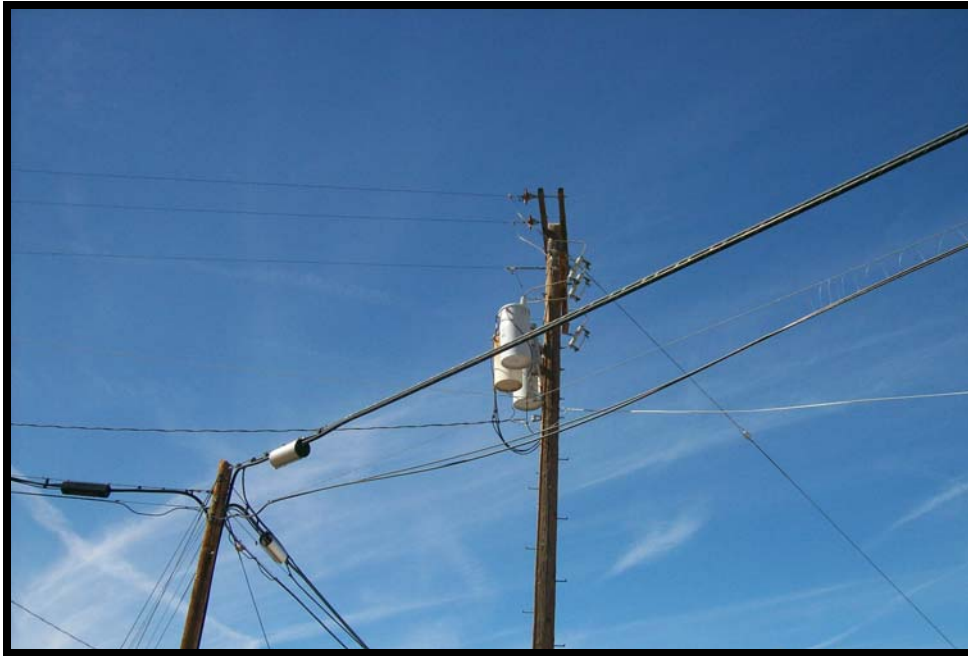
Photograph 15: View of pole-mounted transformer on western portion of subject site.
