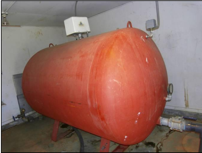
Photograph 53. Interior view of the on-site pump house (pressure tank).
