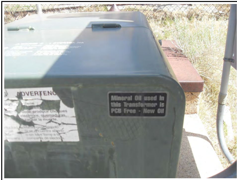
Photograph 25: Pad-mounted transformer PCB-free sticker
