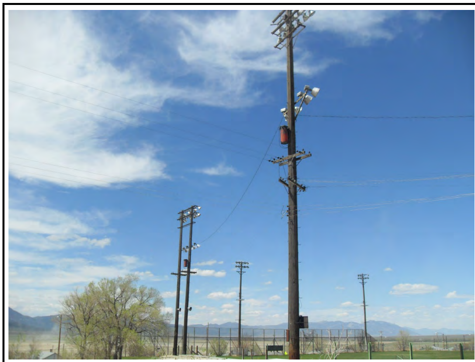
Photograph 26: View of pole-mounted transformers
