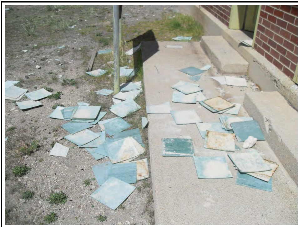
Photograph 29: View of scattered bathroom tiles proximal to bathroom structure
