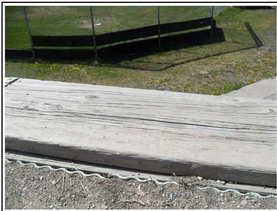
Photograph 22: View of siding on bleachers – below grade
