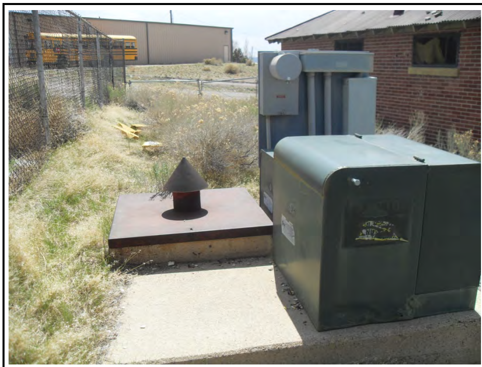
Photograph 24: View of pad-mounted transformers with utility vault venting system
