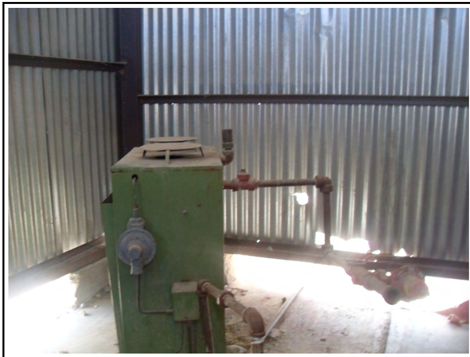
Photograph 31: Propane heater equipment in shed adjacent to bathroom (outside of fenced area)
