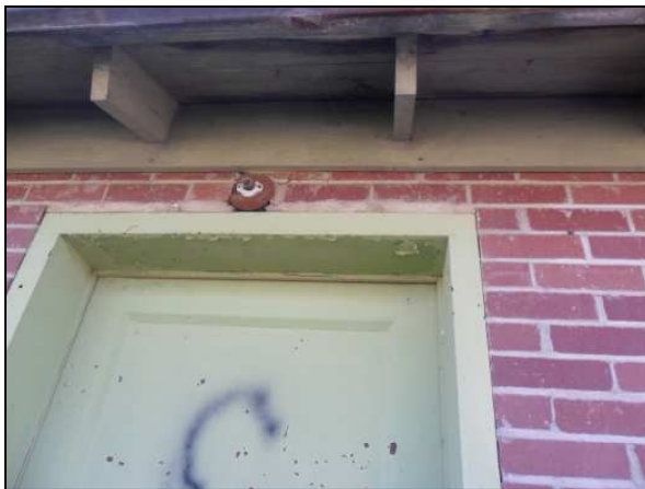
Picture 5 - Exterior Door, Doorframe, Fascia and Joists on the Restroom Building.
