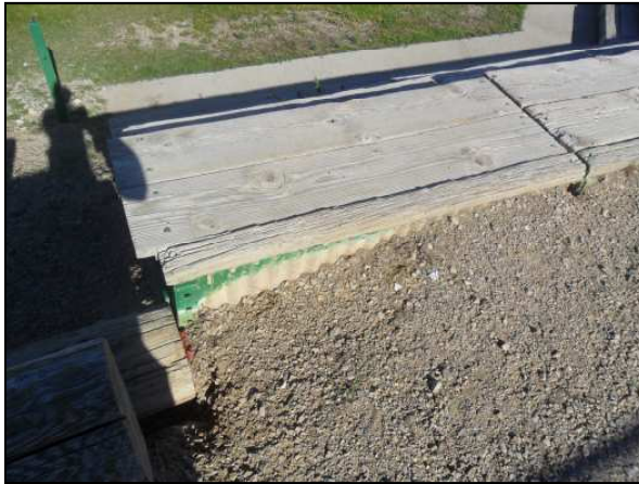
Picture 3 - Corrugated Transite Siding Behind the Outfield Bleachers. (From Above)
