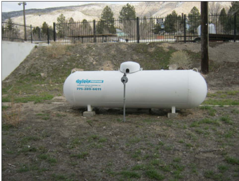
View of a 350 gallon propane AST for heating supplied by Suburban Gas looking east
