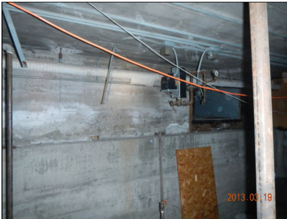
View of a basement pipe - may contain suspect ACM
