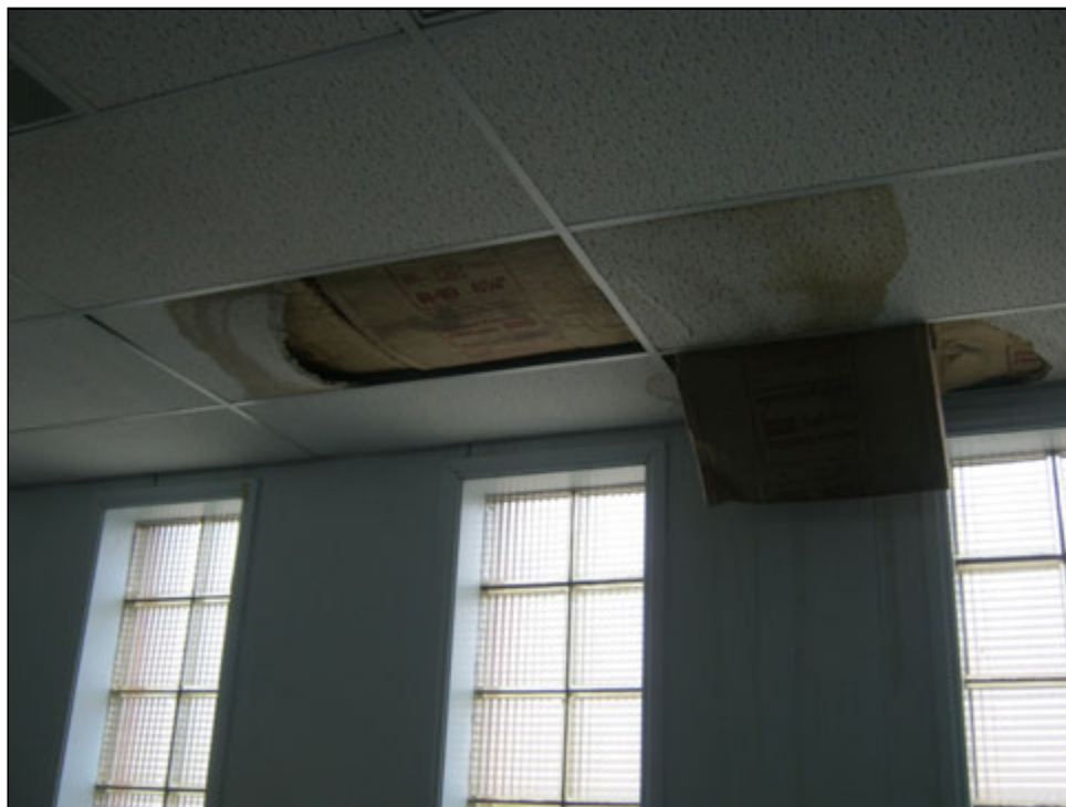
View of water damage on the ceiling tiles within interior of the building
