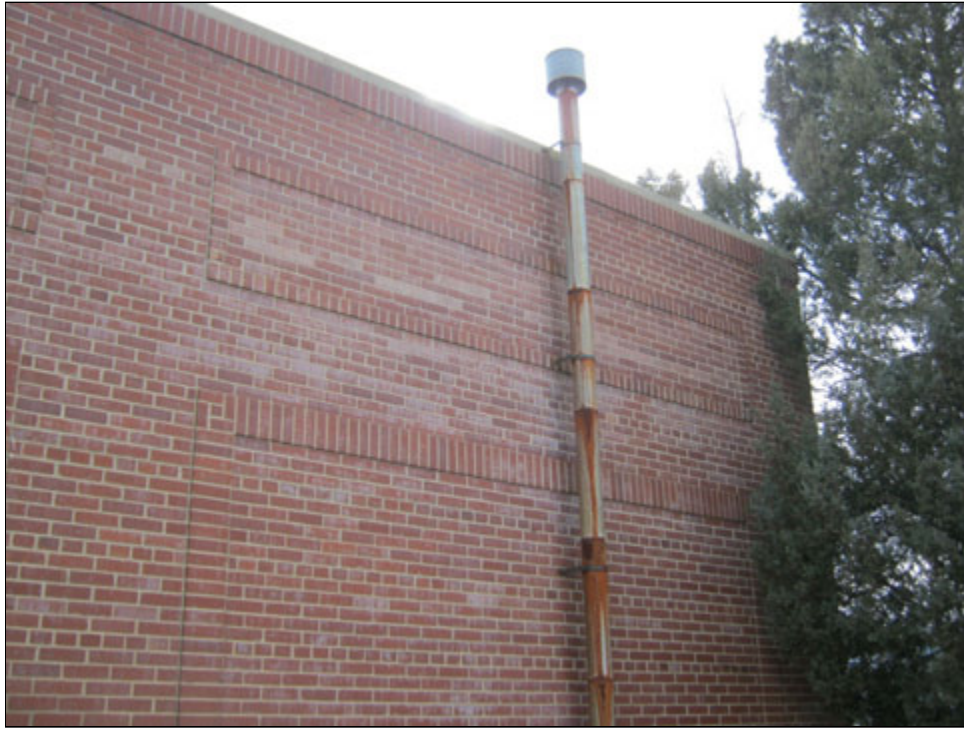
View of heat dissipating vent pipe utilized by former boiler and is no longer in use
