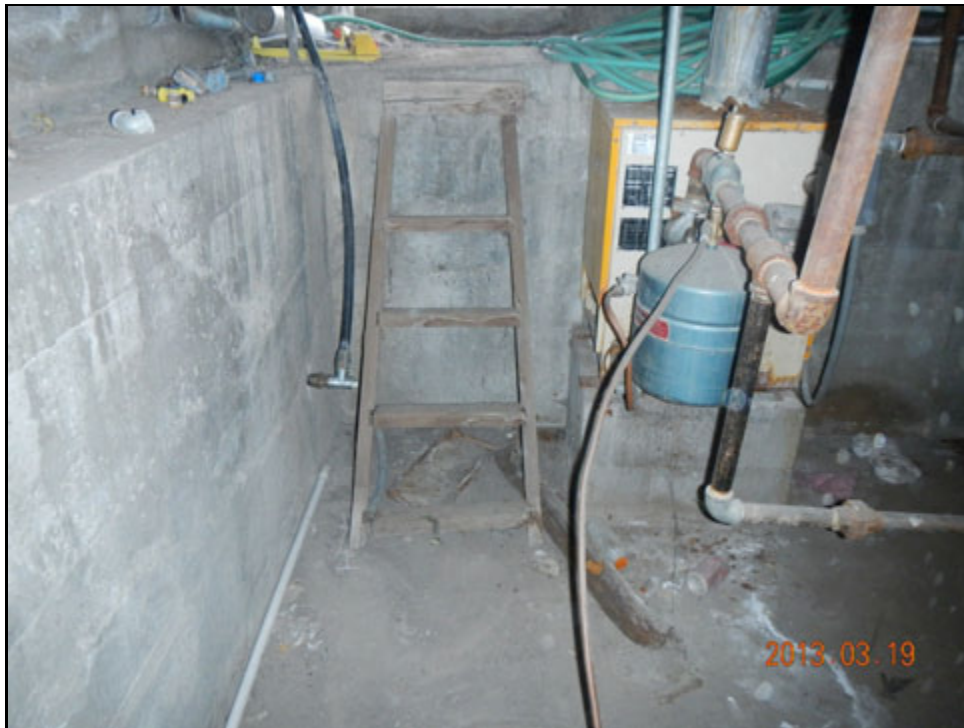
View of domestic water pipe and a former boiler that is no longer in use
