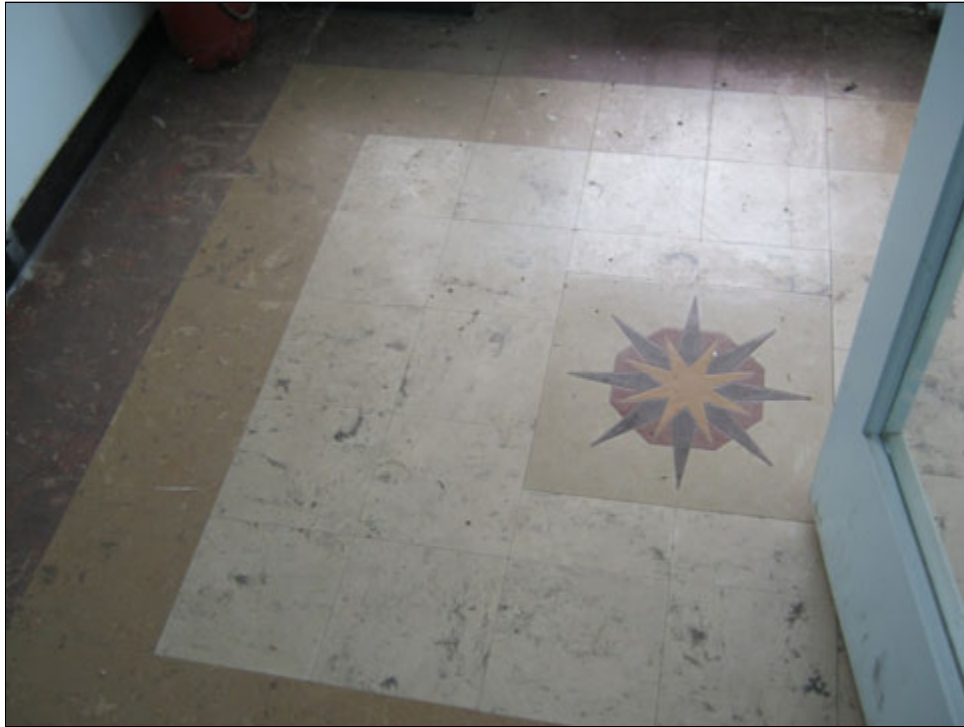
View of tiles in the entrance that may potentially contain ACM
