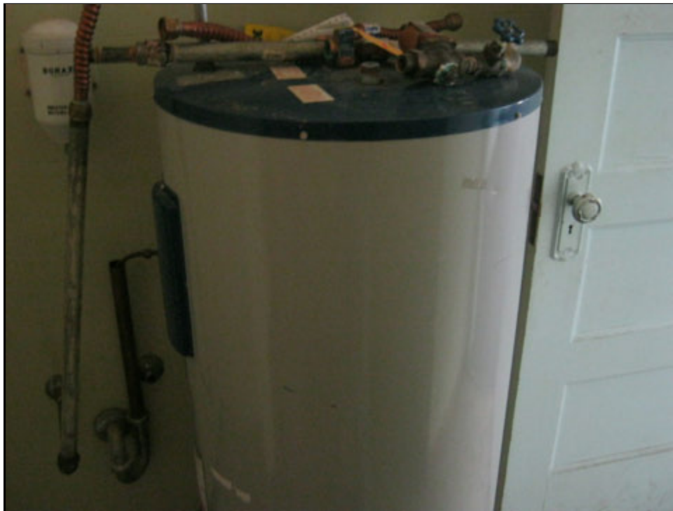
View of a 50 gallon hot water tank in the utility room
