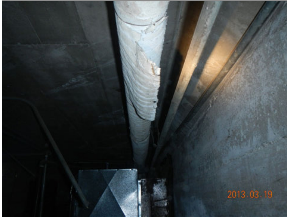
Looking at a pipe with friable insulation that may potentially contain ACM
