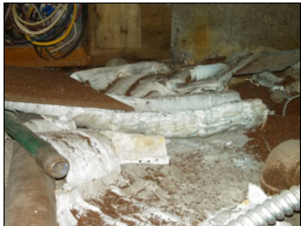
Picture 6—Asbestos containing TSI debris in the northwest basement.
