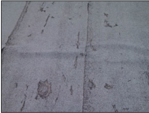
Picture 1—Heavily worn and bucking asphalt roll roofing above the southeast section of the main room.
