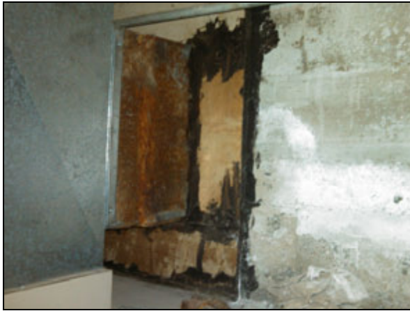
Picture 7—Asbestos containing black wall mastic in the northwest basement.
