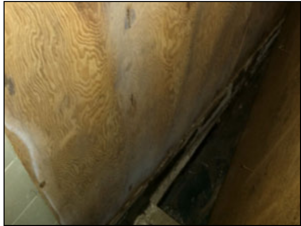
Picture 4—Water damaged plywood behind the paneling on the north wall in the men's room.
