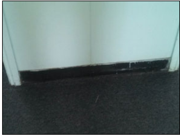
Picture 2—Asbestos containing black vinyl base cove on the wall in the main room.
