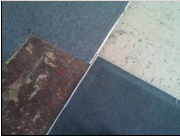
Picture 1—Asbestos containing 9"x9" VCT (including beneath carpet) on the floor in the main room.
