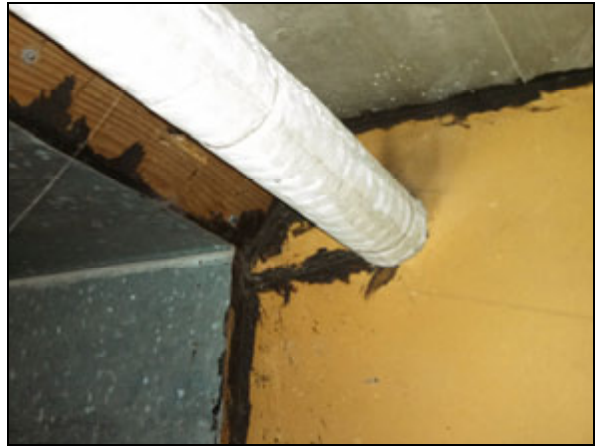
Picture 8—Asbestos containing TSI and black wall mastic in the northwest basement.
