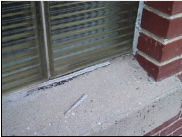
Picture 3—Asbestos containing white window putty around the perimeter of the block windows on the east side of the building.
