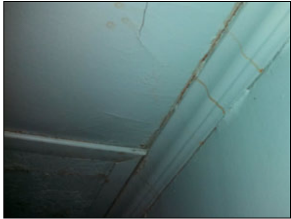
Picture 2—Water damaged wall, ceiling, and crown molding above the drop ceiling in the southeast section of the main room.
