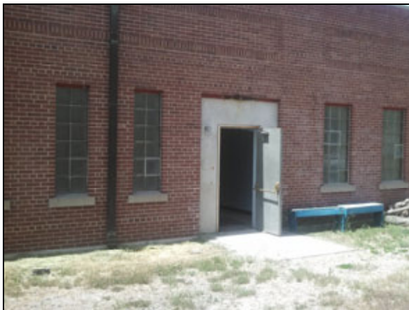
Picture 11—East side of the building showing the gutter downspout with leaded solder and block windows with asbestos containing putty.
