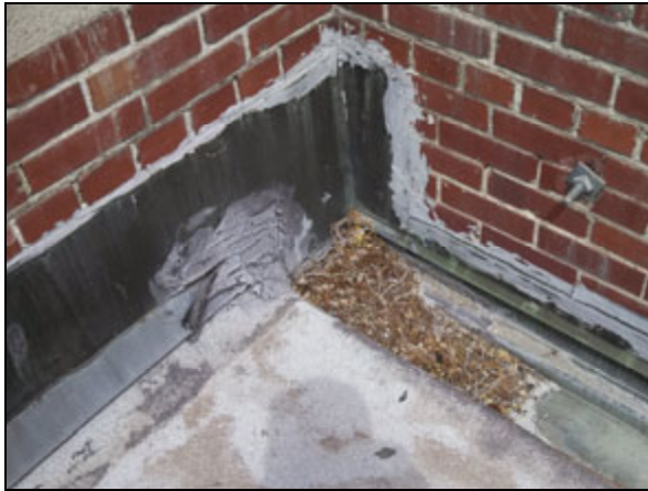
Picture 3—Old roof mastic used to seal seams on and adjacent the metal gutter. Note that the gutter is on the interior of the building's outer brick wall.
