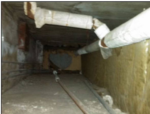
Picture 5—Asbestos containing TSI on the pipes in the north crawl space beneath the building.
