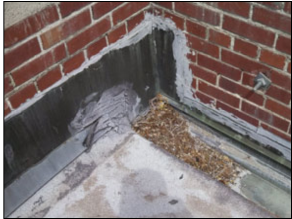
Picture 4—Asbestos containing gray roof mastic on the main roof.
