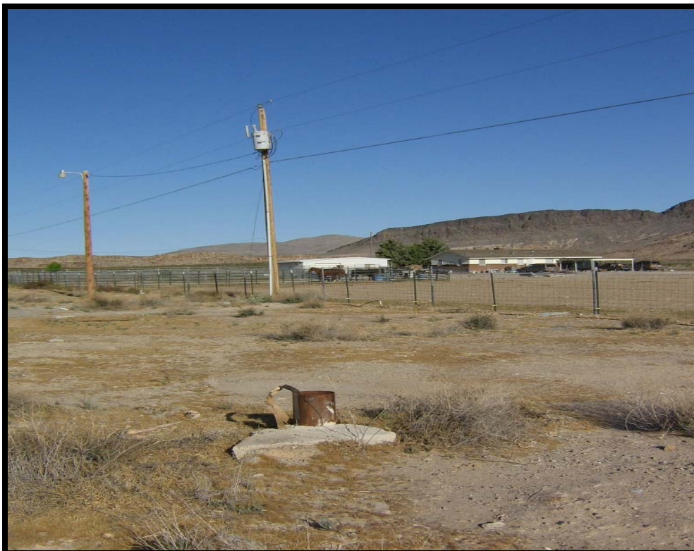
Photograph 6: View of well casing and pole-mounted transformer on northern margin of site, facing northwest
