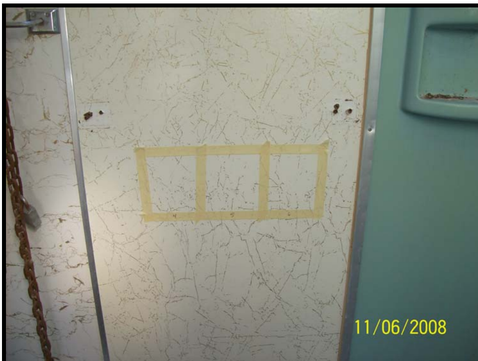
Photograph 2: View of surface wipe sample locations BTR1-SWP-4M, BTR1-SWP-5L, and BTR1-SWP-6I in bathroom.
