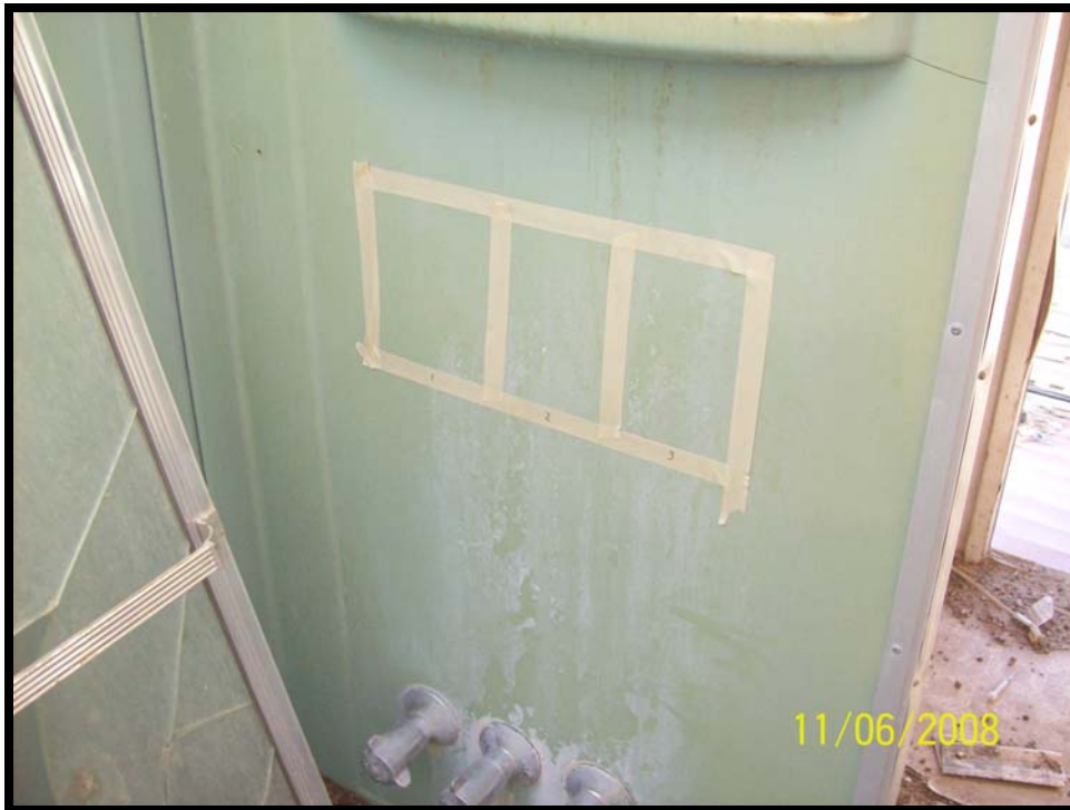
Photograph 1: View of surface wipe sample locations BTR1-SWP-1M, BTR1-SWP-2L, and BTR1-SWP-3I in bathroom.
