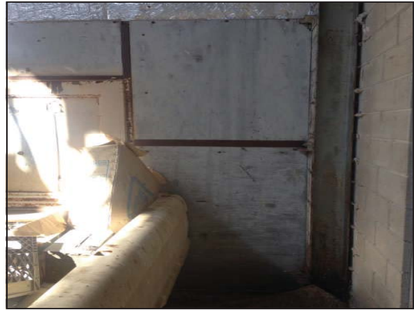
Picture 20—Gray wood wall found in the open room in the fabrication building.
