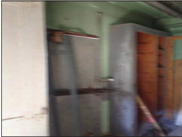
Picture 21—Green wood wall found only in room 1 in the fabrication building.
