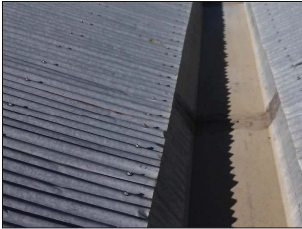
Picture 7—Roof mastic in the center gutter on the roof of the fabrication building.
