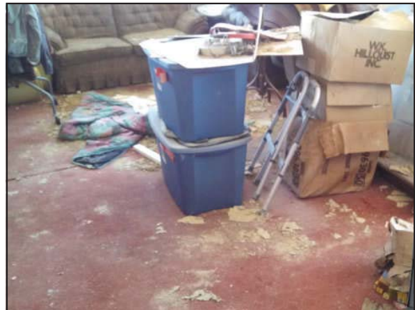
Picture 4—Acoustic ceiling debris on the contents and carpet in room 1 in the second floor of the house.
