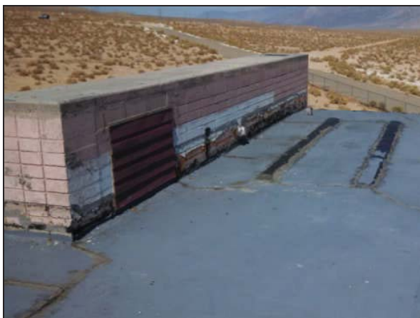
Picture 5—Gray roof mastic on the cracks and parapet wall on the roof of the house.
