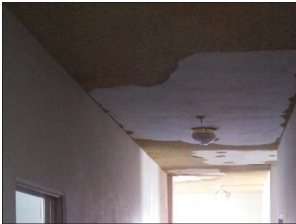
Picture 1—Damaged acoustic ceiling texture in the second floor hall in the house.
