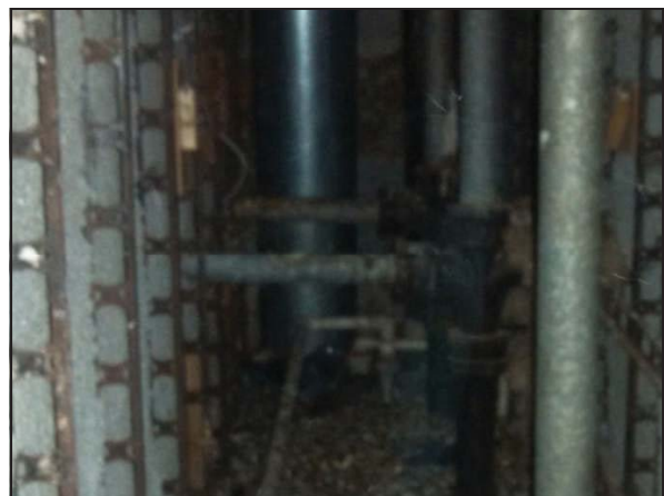
Picture 6—No suspect asbestos containing materials in the chase behind the bathroom wall.
