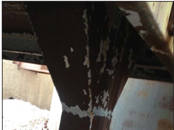
Picture 34—Yellow and gray metal ducts and framing of the elevator system adjacent the silos.
