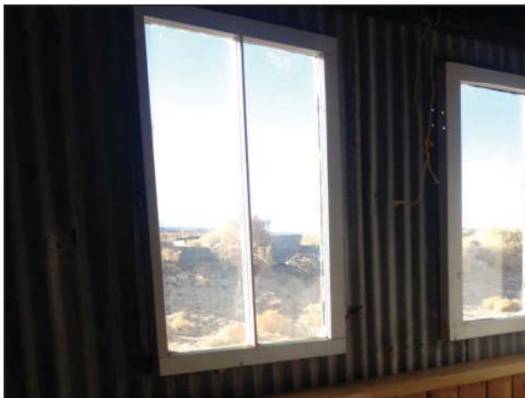
Picture 29—White wood window frames on the west side of the mill.
