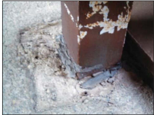
Picture 16—Mastic beneath center silo and above the basement beneath the silos.
