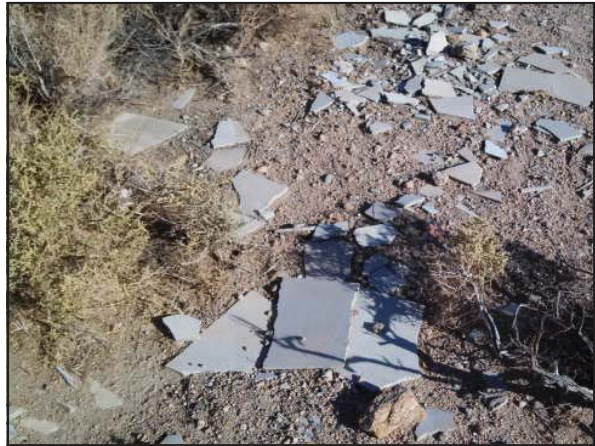
Picture 10—Broken cementitious panels directly adjacent to the collapsed building.
