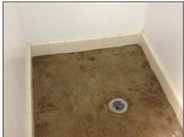
Picture 30—White ceramic baseboard tile in the shower of the new bathroom in the mill.
