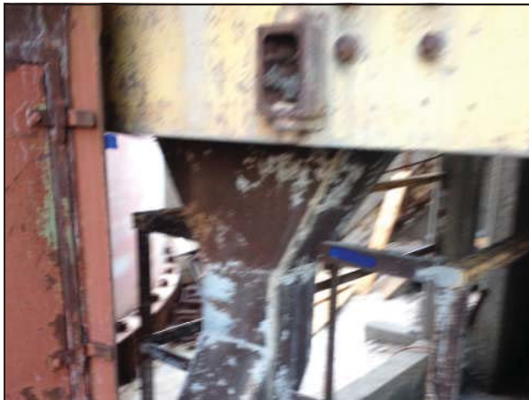
Picture 33—Yellow and gray metal ducts and framing of the elevator system adjacent the silos.
