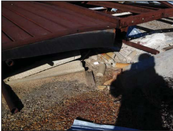
Picture 9—Damaged TSI amongst the debris of the collapsed building.
