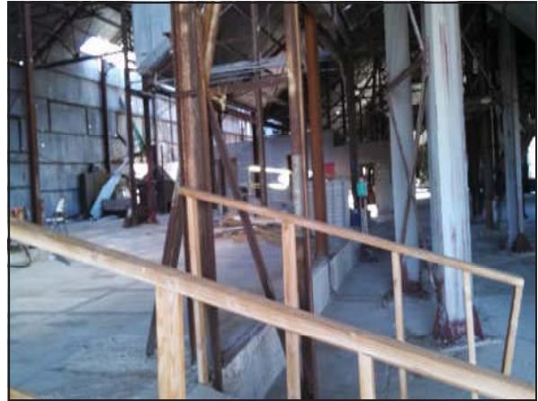
Picture 28—Gray, red and brown metal framing and hopper supports found in the mill.
