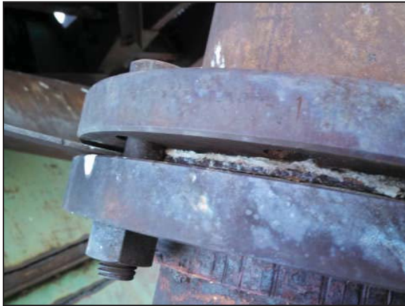
Picture 15—Gasket at pipe junction above the center silo.
