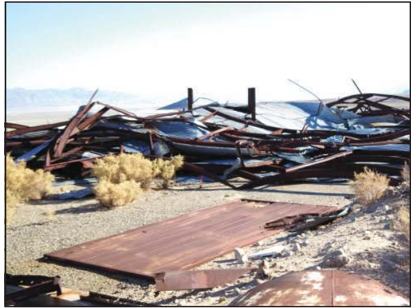
Picture 8—Collapsed building in the southeast corner of the property.
