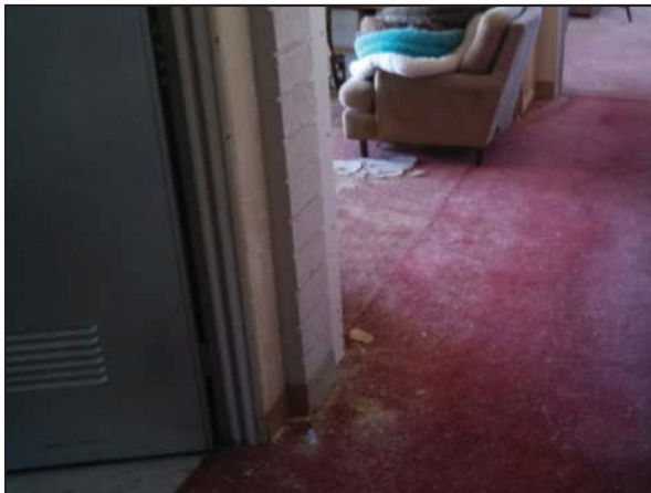
Picture 3—Acoustic ceiling debris on the carpet in the second floor hall in the house.
