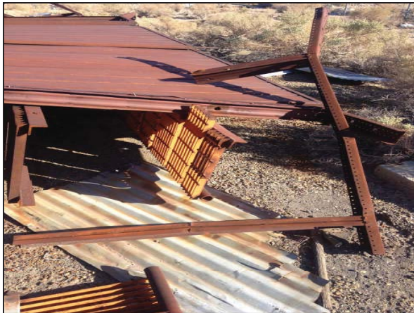
Picture 23—Orange grates found in the collapsed building.
