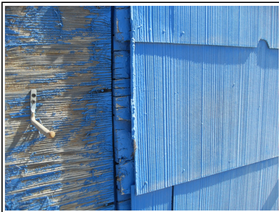
Photograph 22: View of exterior transite siding and flaking paint
