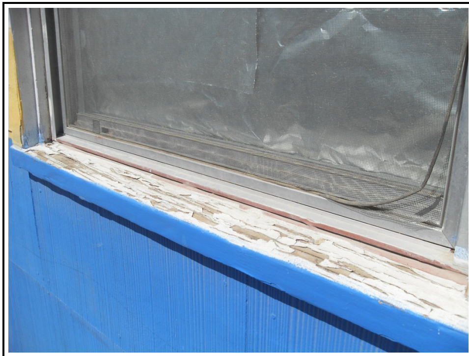
Photograph 23: View of flaking exterior window sills
