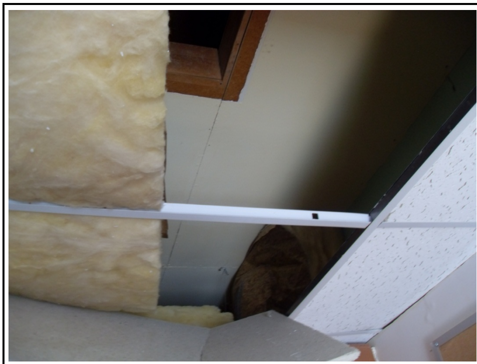
Photograph 12: View of original ceiling above drop down in sports equipment storage room
