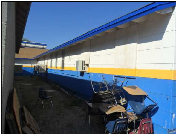
Picture 5 - Exterior Transite Walls, Window Frames, Window Sills, Soffits and Joists on the West Side of the Building.
