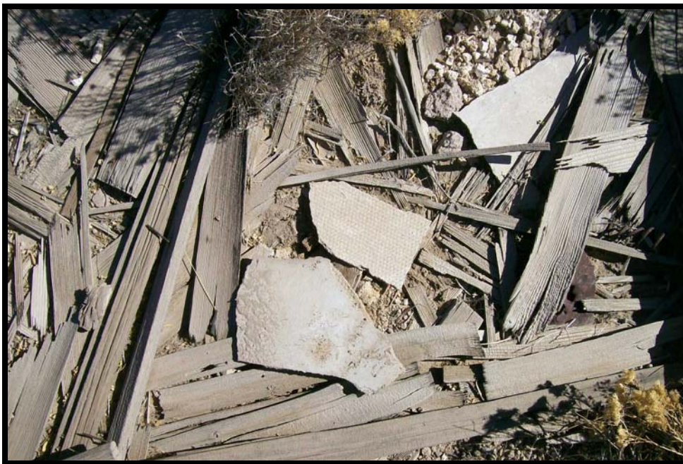
Photograph 12: View of transite paneling on subject site.
