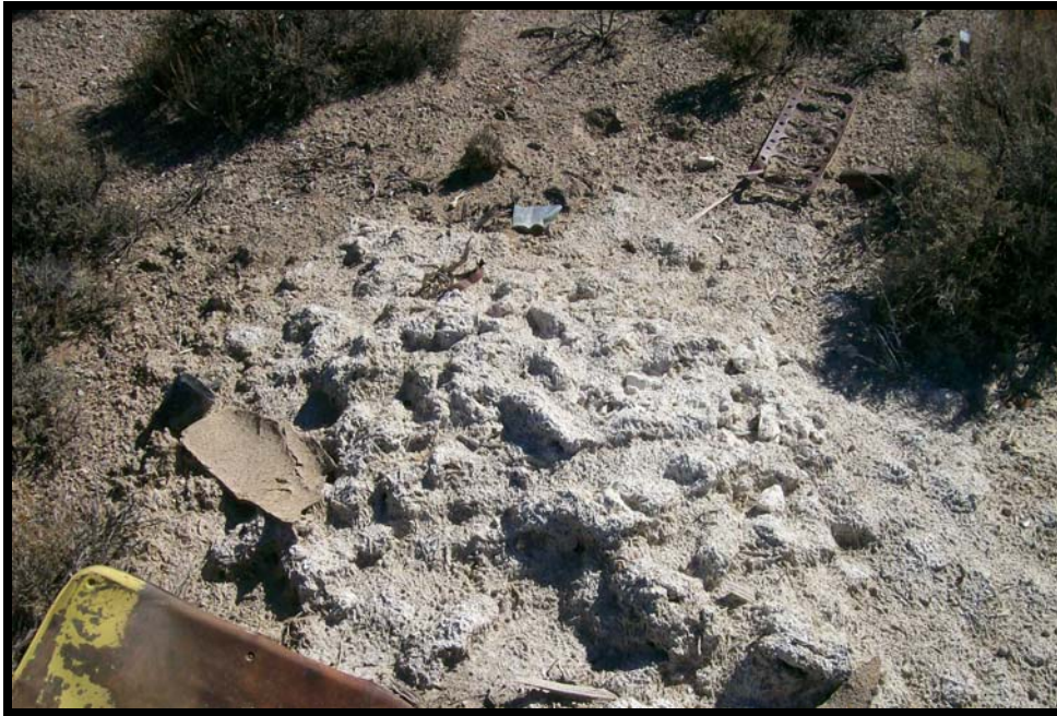
Photograph 15: View of thermal systems insulation on subject site.
