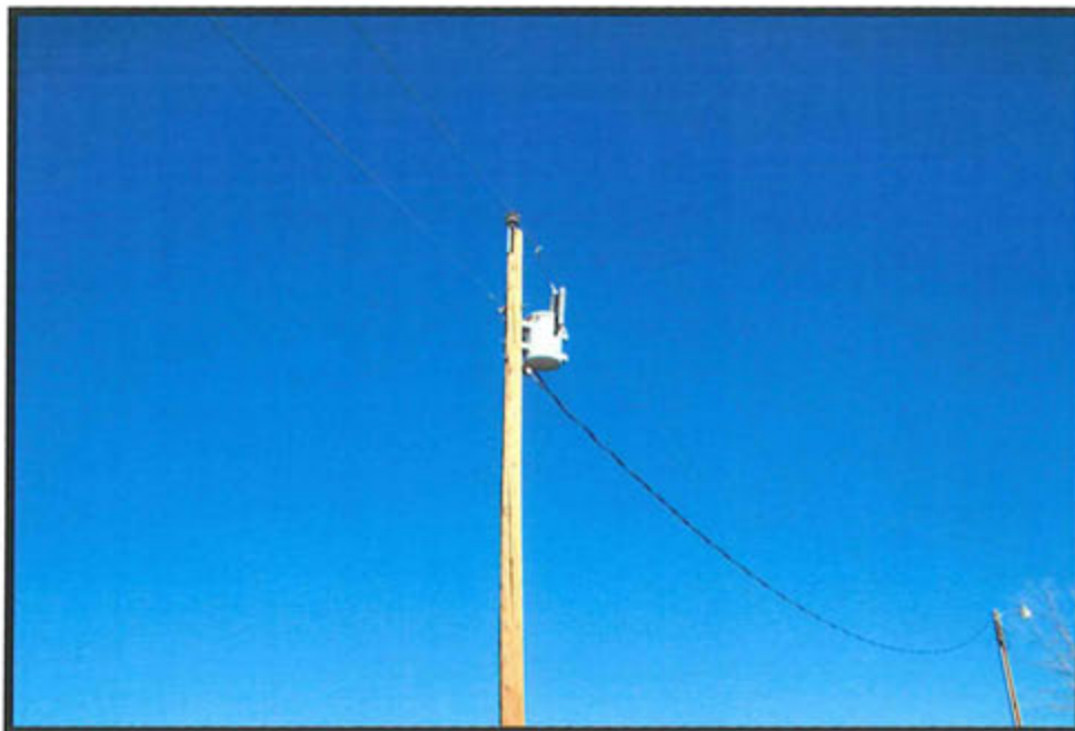
Photograph 18: View of pole-mounted transformer, facing northeast.
