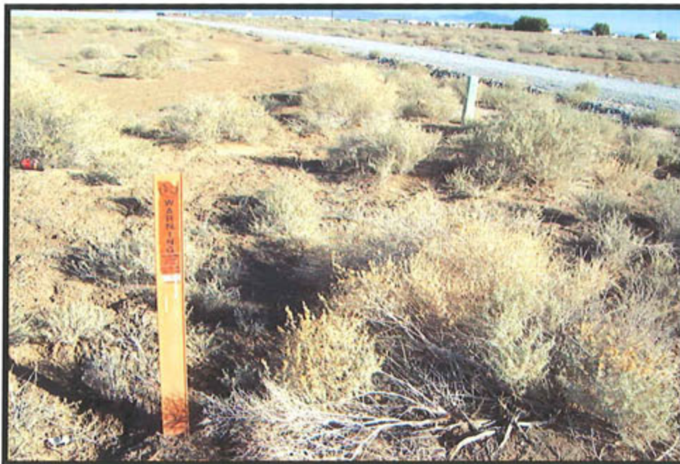
Photograph 16: View of utility warning marker and utility box located near southwest corner of subject site, facing southeast.
