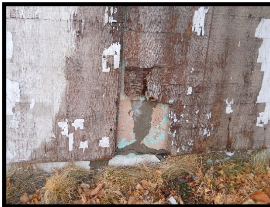
Photograph 7: Exterior of FBO building documenting representative section of concrete / wood-panel wall extremely weathered condition. (looking west).
