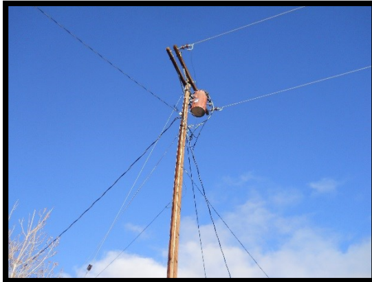
Photograph 9: Pole mounted transformer on the northwest corner of site (looking east).
