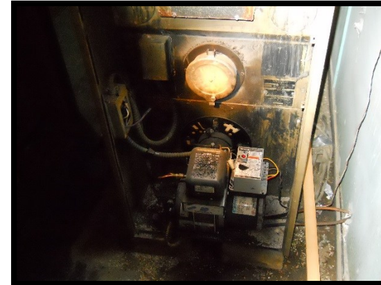
Photograph 10: Fuel fed furnace housed within active FBO building.
