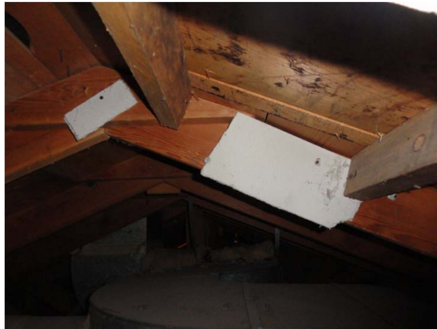
Remnant Transite Wallboard in Attic
