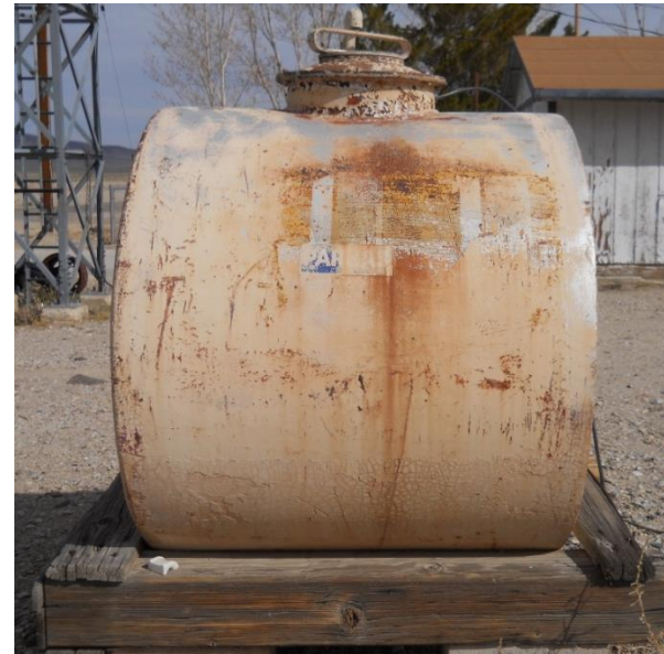
Photograph 2: Above ground storage tank (facing north)
